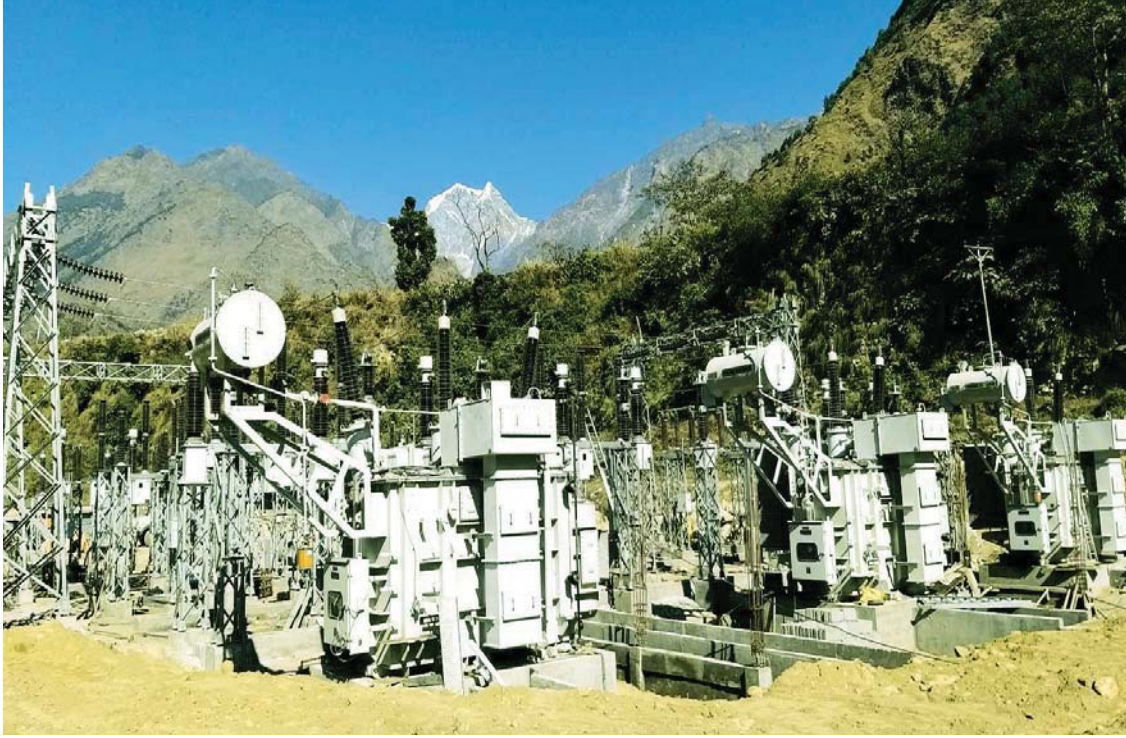
MISTRI KHOLA HEP SWITCHYARD
