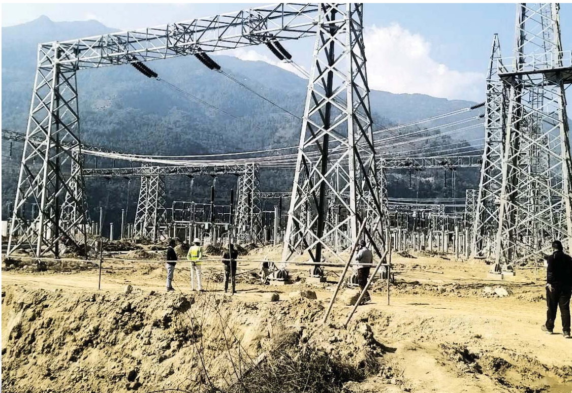
MISTRI KHOLA HEP SWITCHYARD
